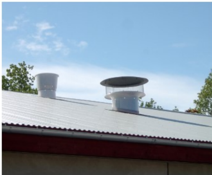
Breeder house with DA 60-820 roof inlet and DA 820 chimney outlet
