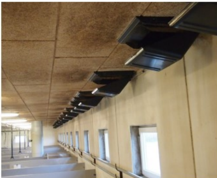
DA 1540 ceiling inlets opened for traditional side mode ventilation. The air adheres to the ceiling before returning in the zone occupied by the animals
