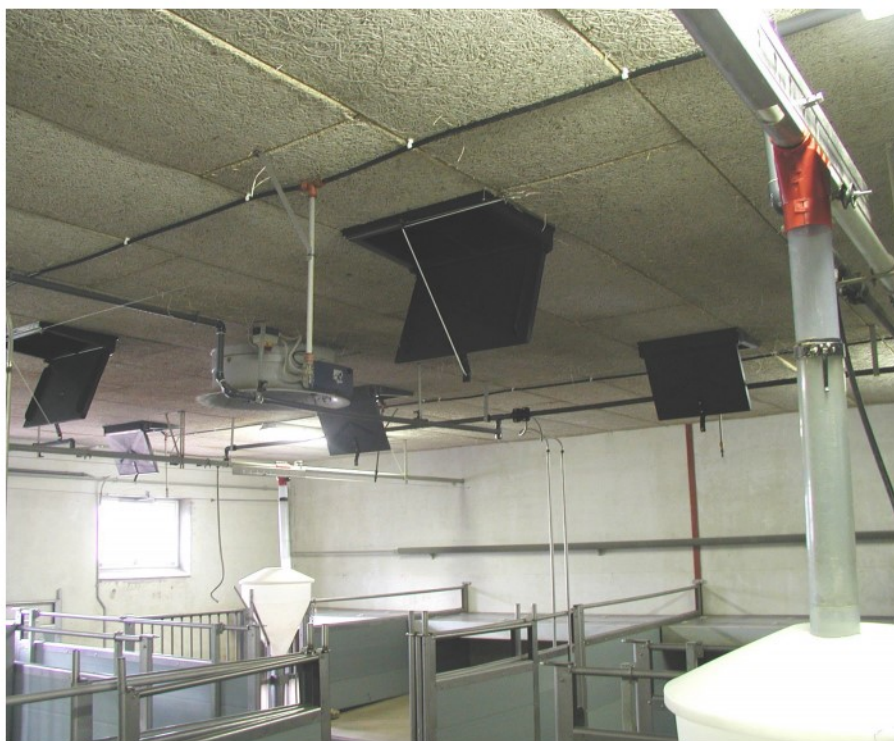
Combi-Diffuse ventilated house with DA 1800 ceiling inlet
