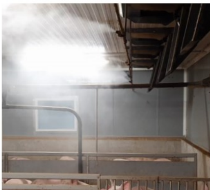
The DA 1540 chill inlet creates a vertical air flow to chill the pigs in the lying area
